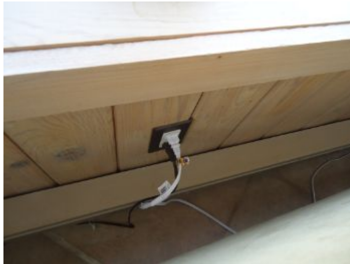
electrical cords too close to heater on porch
