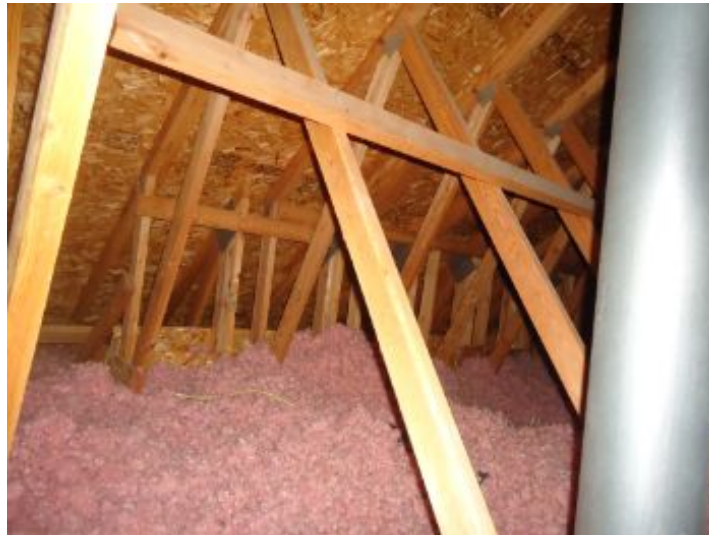
insulation in attic uneven, recommend adding some
