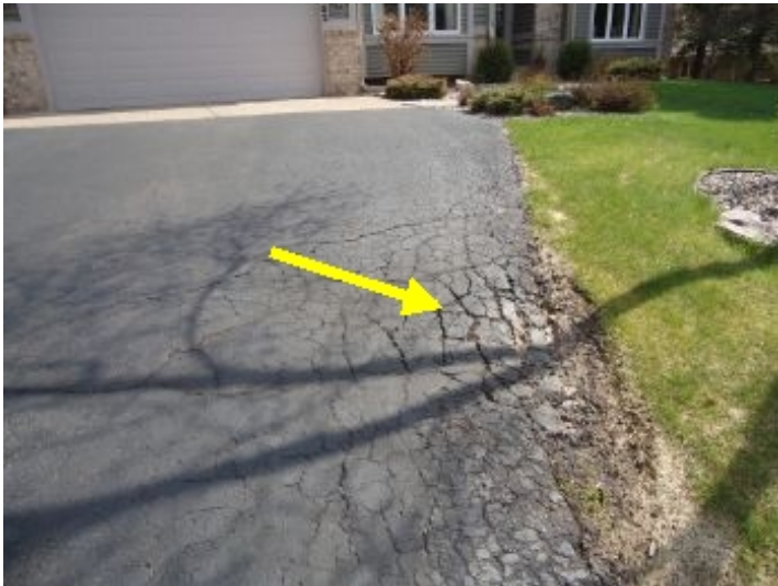
will deteriorate further
