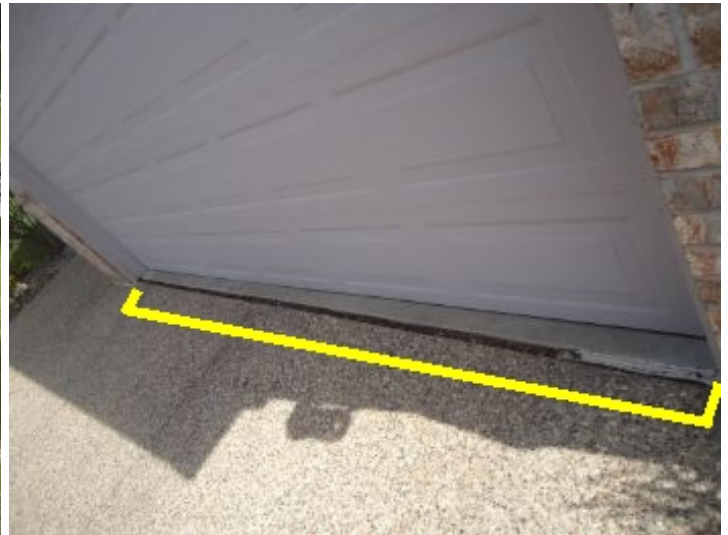
add sealant to gap at garage apron
