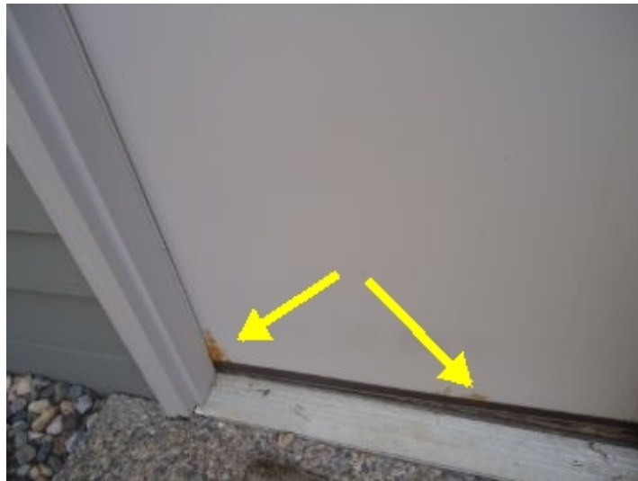
metal garage service door rusting
