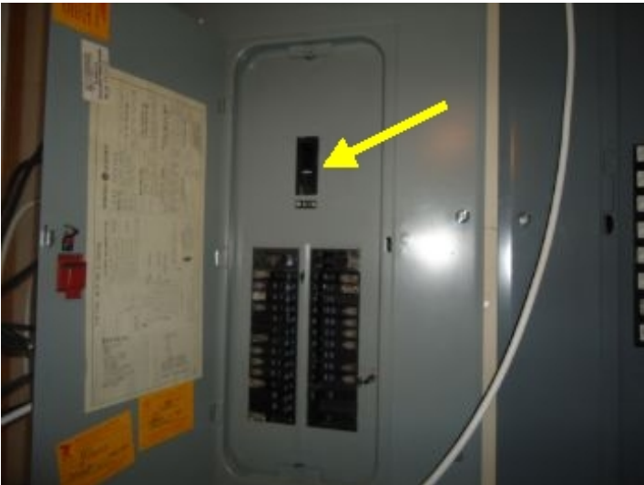
on left hand of two panels, this is main shut off of electric
