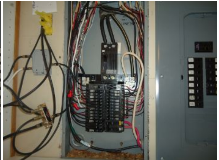
inside of main panel
