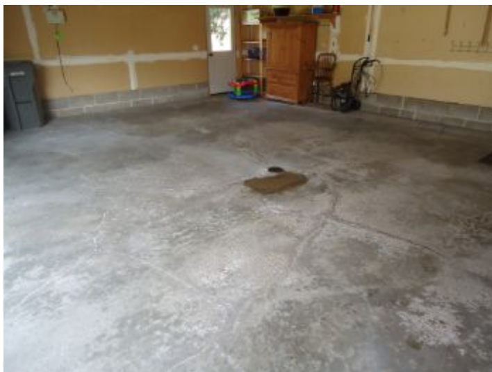
normal, typical concrete cracking in garage floor
