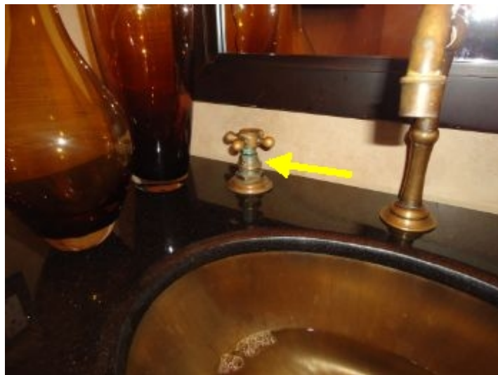
green patina indicates past leak, not presently active
