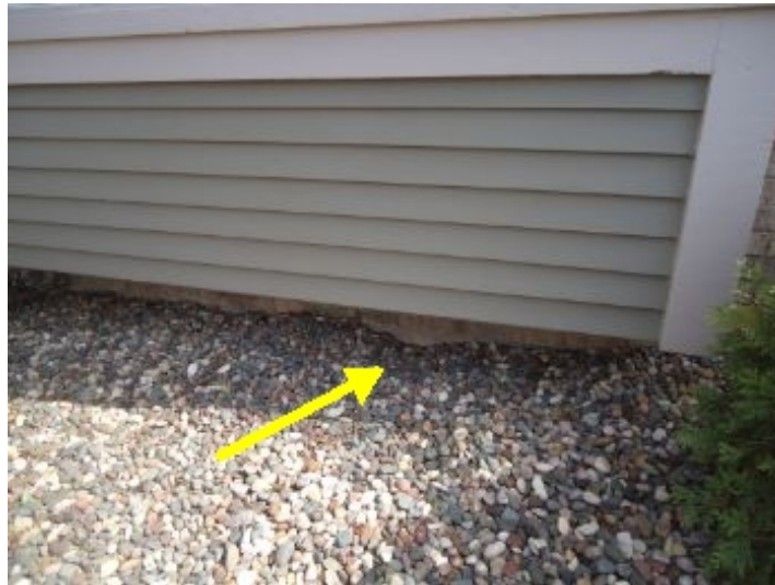
minor settling under bump out on front of house
