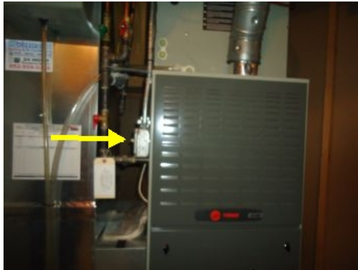
electric shut off switch for furnace
