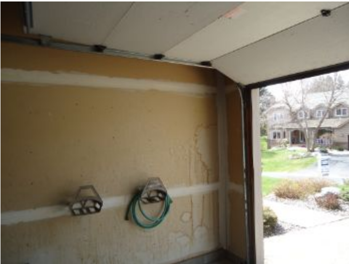
water stains on garage walls
